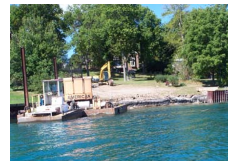
Construction of a new seawall on the St. Clair River in St. Clair Township.
